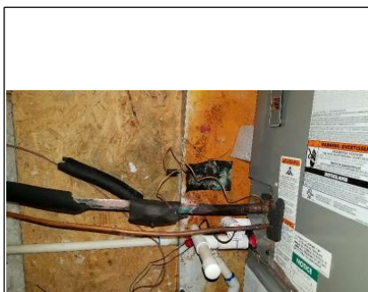
Insulation damaged/missing around heat pump suction line at air handler - recommend repairs or replacement
