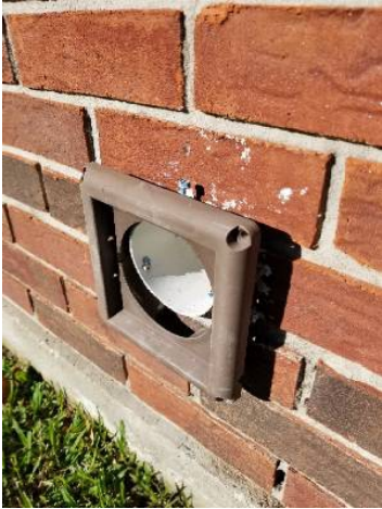
Laundry dryer vent cover at exterior wall damaged/missing - recommend repairs or replacement
