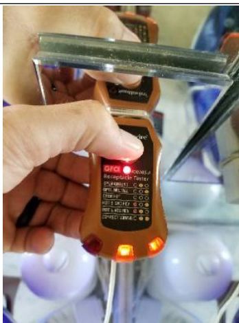
All outlets located in bathrooms should be GFCI protected - recommend upgrading outlets for GFCI protection
