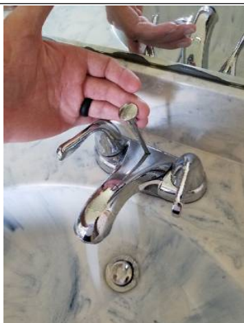
Drain stop in master bathroom not operating properly during time of inspection - recommend repairs or replacement
