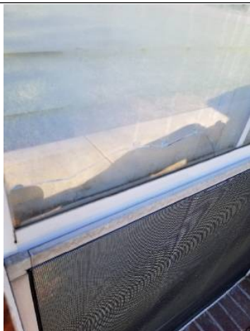
Cracked window noted at front side of home during time of inspection - recommend repairs or replacement
