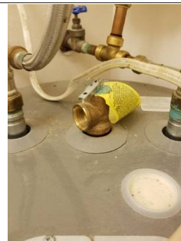
Water heater missing TPR valve discharge pipe - Temperature-Pressure Relief valve extension pipe should extend to within 4"-6" off of the floor - this is a Safety Concern - recommend repairs
